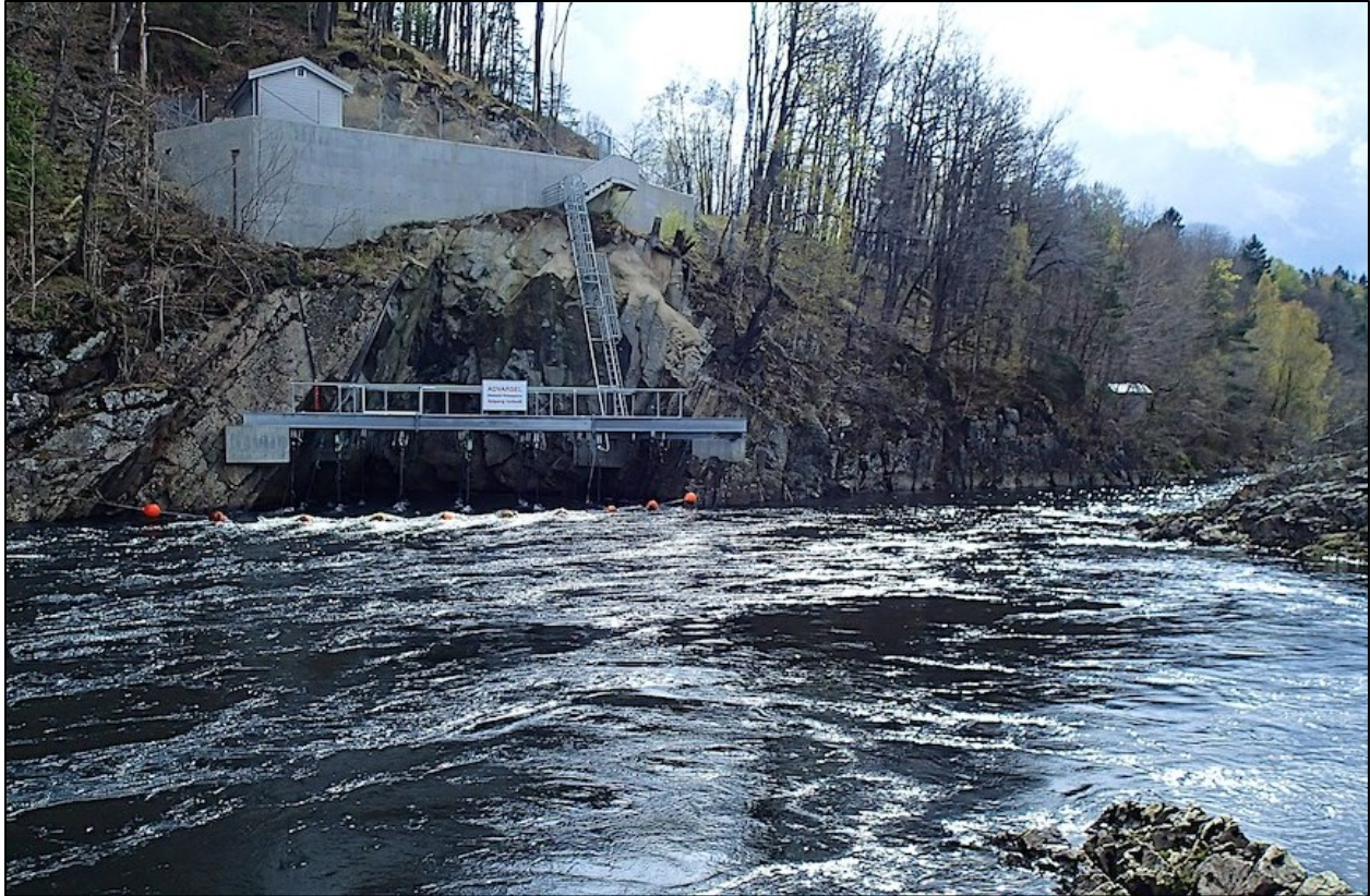
Figure 5. The electrical barrier at the outlet of the Rygene Power Plant power tunnel on Nidelva in southern Norway. Three vertical rows of electrode cables are affixed to the overhead steel structure and the tunnel floor, presenting the electrical deterrent field uniformly at all depths in the water column. The barrier has been demonstrated to successfully deter anadromous fish from migrating upstream in the power tunnel, allowing them to continue their upstream migration in the river channel.
